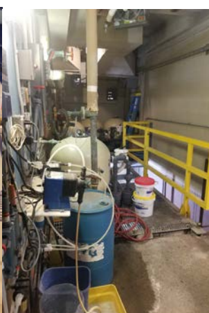
Panzer Gym Pool Control Room
